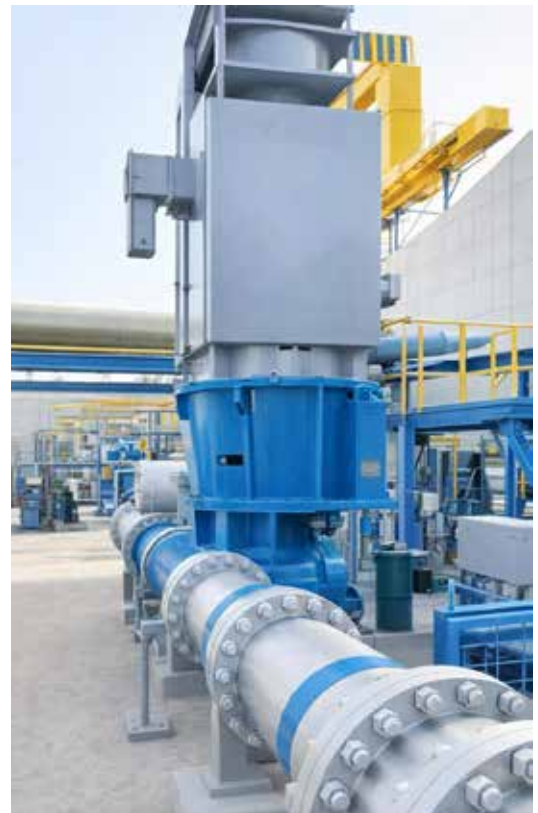
A DD-V pump installed at Power and Desalination plant
