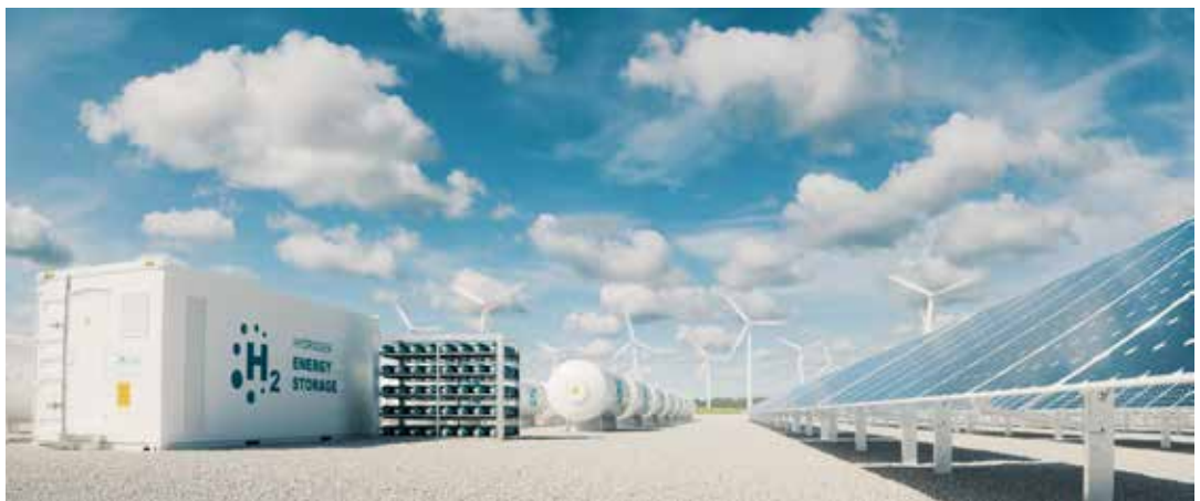
Hydrogen is important in the transition to renewable energies
