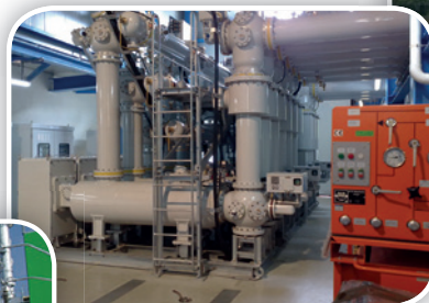
150kV GIS Belgium
