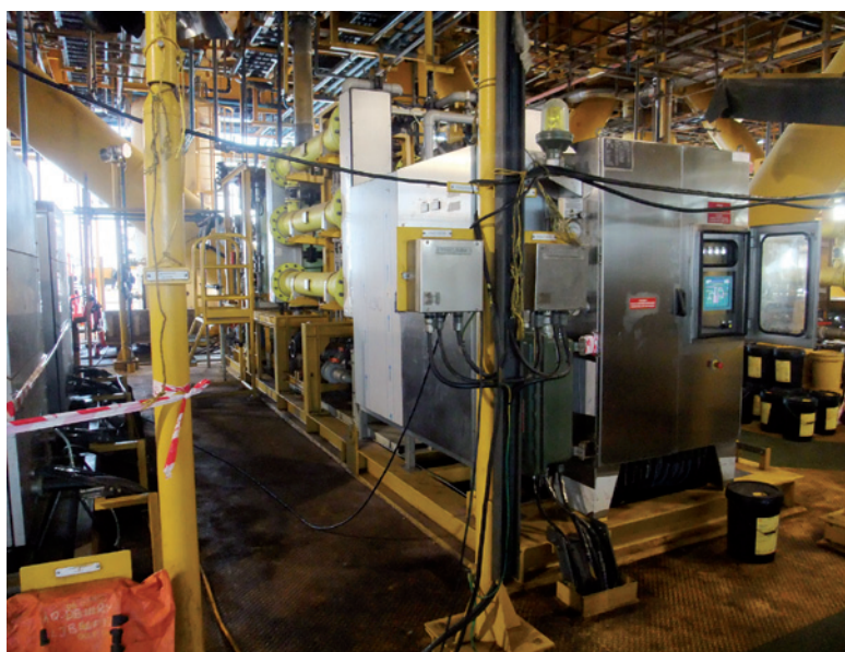
Fig. 2 - The electrochlorination package working on platform
