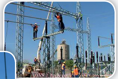
110kV AIS Mozambique
