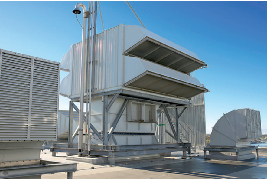
Fig. 1 - Air Inlet System for a Siemens SGT800 gas turbine (courtesy Camfil Power Systems)
