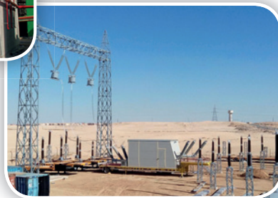
400/220kV Mobile Algeria
