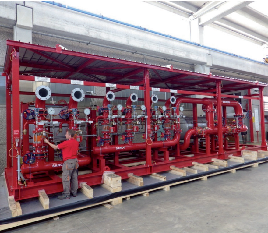
Fig. 2 - Deluge valves on skid
