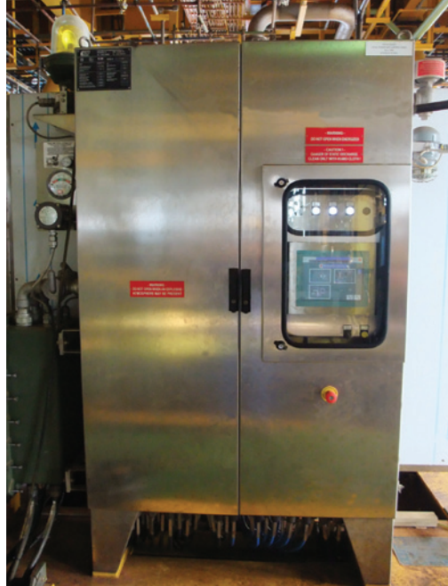
Fig. 3 - Ex p power & control panel
