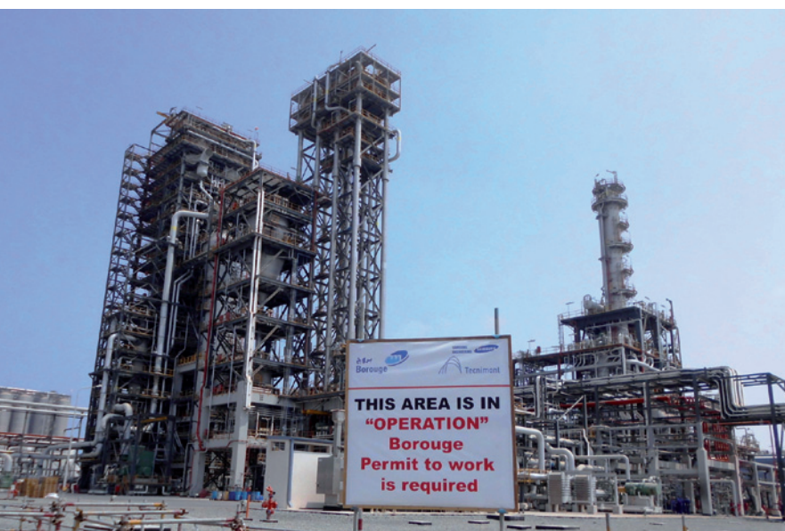
Fig. 2 – Polyethylene loop and gas phase reactors
