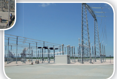
400kV AIS Italy
