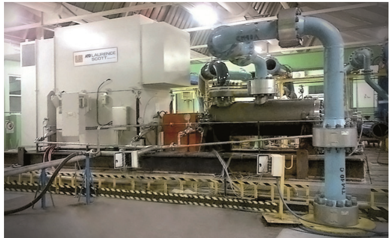
Fig. 4 - Testing the 5,6 MW Water Injection Pump Unit in Sesto San Giovanni facility
