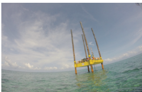
Fig. 2 - Near shore Geotechnical site investigation - Jack up rig performing Boreholes and Piezocone Penetration Tests (PCPT)
