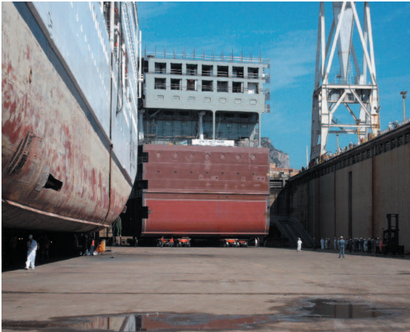
[Figure 11.1 – Skidding of half ship and transport of new ship section for MSC Fin-cantieri Jumboization Project]
