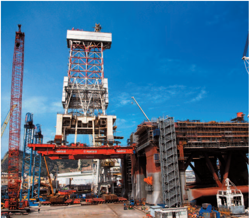
[Figure 8.5 – Drilling Tower Module lifting and skidding with elevator system for Scarabeo 8 Saipem Platform in Fincantieri Palermo (Fagioli)]
