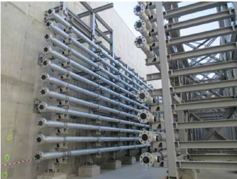
Fig. 8 - Reactor bay with HP reactor pipes
