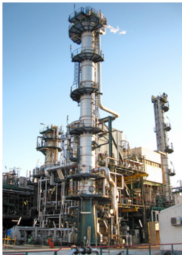
Sour Water Stripper Unit
