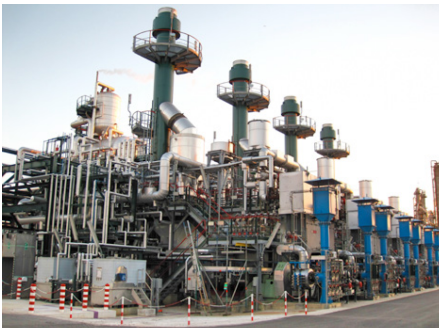
High-Pressure Steam Boilers Unit
