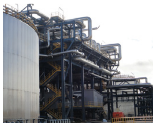
ET Sun Energy™ Thermal Energy Storage for Andasol III Solar Power Plant _ Spain
