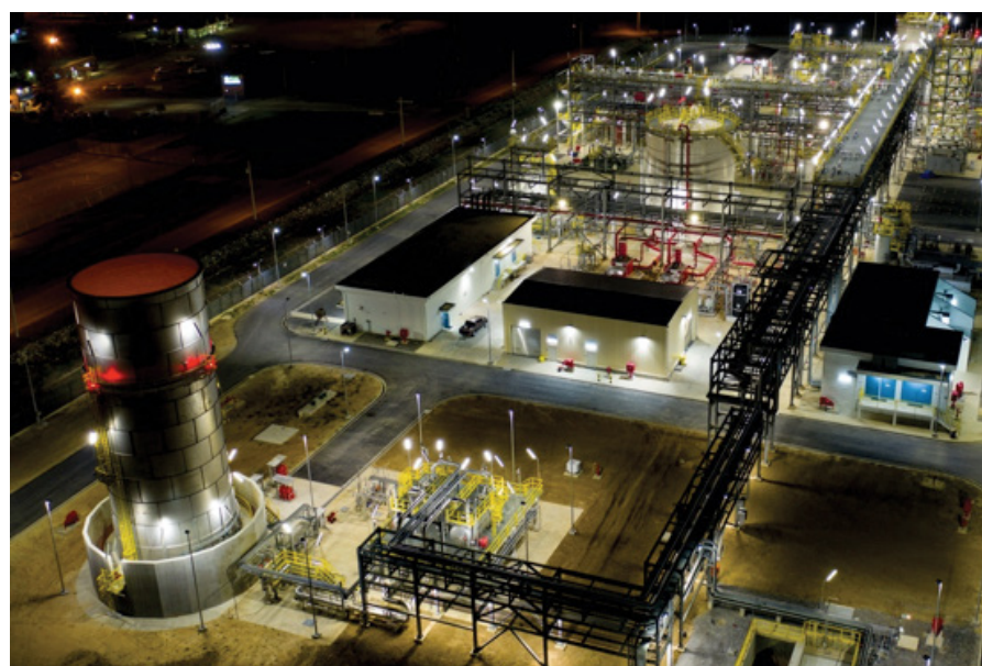
Point Lisas, Trinidad & Tobago – Gas Processing Unit for Denovo Energy
